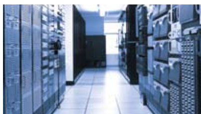
DATACENTER and IT
